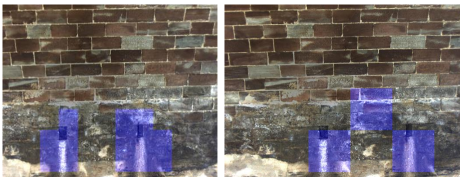
Figure 21: Water leak detection (in blue) in images of a masonry tunnel
