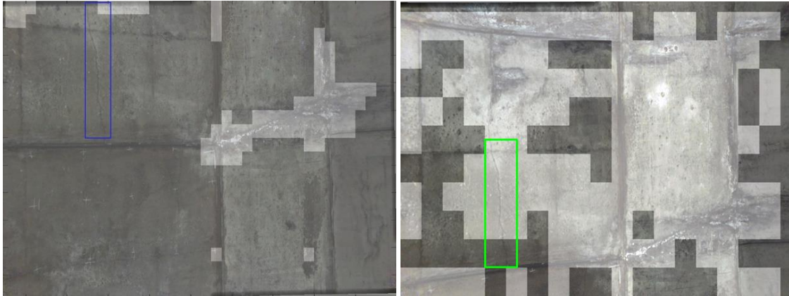
Figure 22: Defect detection (light areas) in concrete tunnel images. Example of a non-detected crack (blue box, left image). The same crack is detected using a more specific training (green box, right image) at the expense of a high rate of false alarms.
