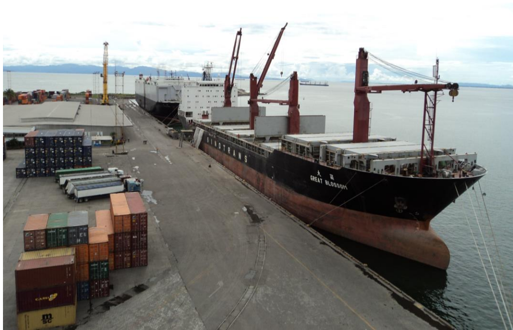
Fig. 11 Quay wall at Puerto Caldera, taken from the end of Berth N.3.
