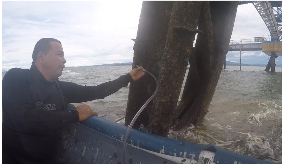
Fig. 19 Thickness measurement in one pile of the first support from the pier
