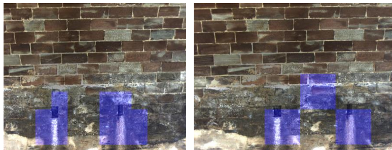
Figure 3: Water leak detection (in blue) in images of a masonry tunnel
