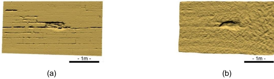
Figure 1: Views of a lack of rubble stone on laser (a) and sonar (b) models of a canal wall
